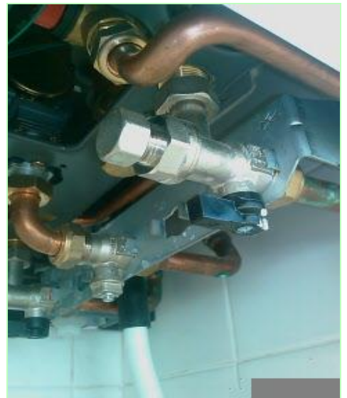
Main heating system
