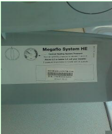
Main heating system
