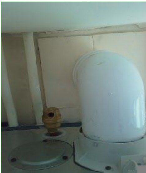
Main heating system
