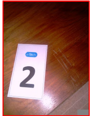
Wooden flooring in Room Floor - scratched (as photographed), Floor - marked
