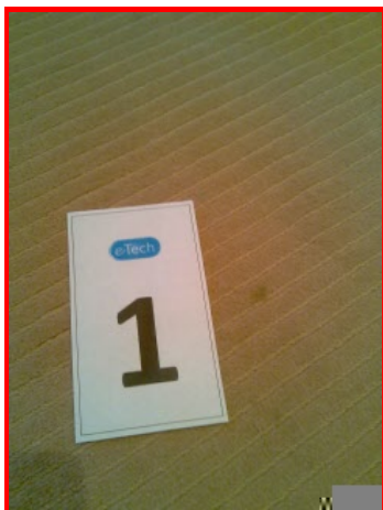
Carpet areas in Room Floor - discoloured (as photographed)
