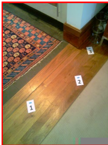
Wooden flooring in Room Floor - scratched (as photographed)
