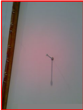
All Walls in Room Wall Finish - hole (nail)
