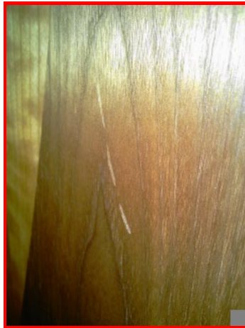
Door to Sitting Room Door Finish - scratched
